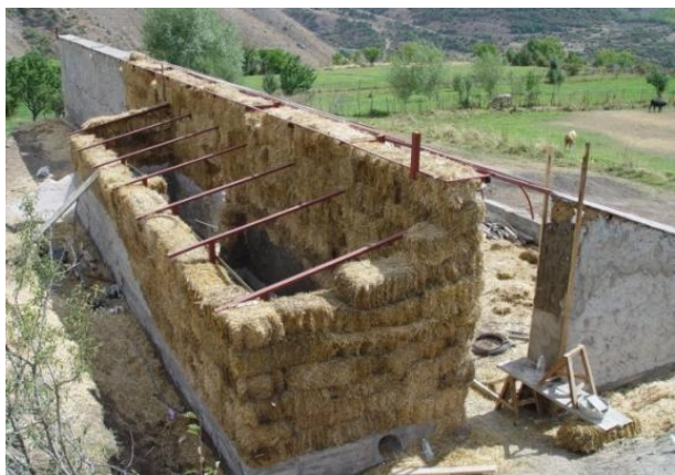
Picture 3. PSG in Horbategh village, Vayots Dzor region. Picture taken during construction, 2015.
